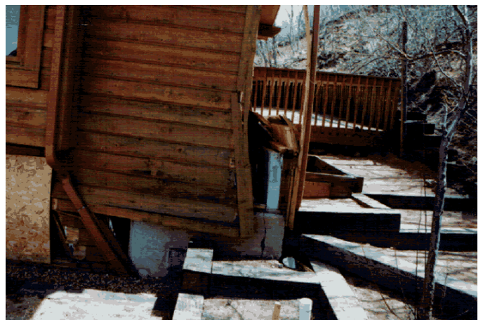
The Garrison residence, a 1996-house ripped from its foundations and condemned. Photo courtesy of John Himmelreich
